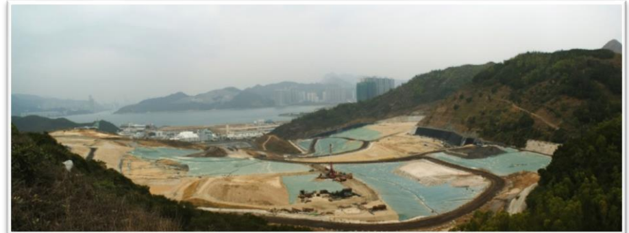
Landfill Gas Utilization
