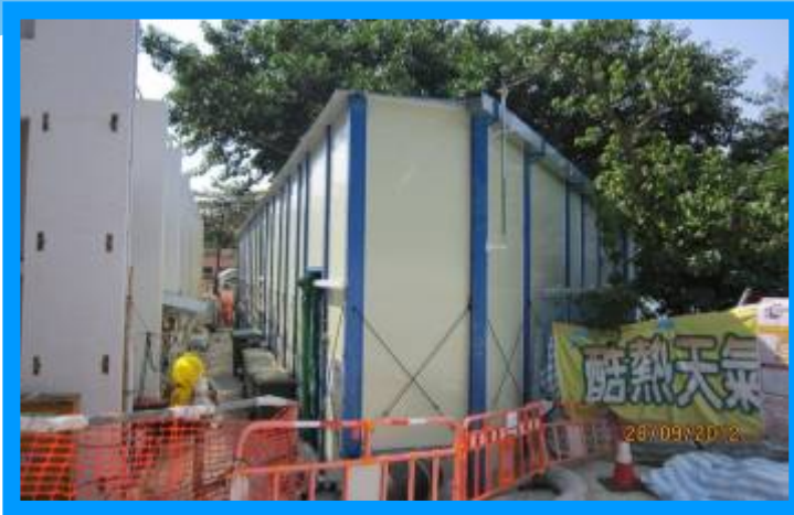
Enclosure for temporary Sewage Treatment Facilities at Wah Fu PTW
