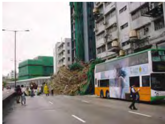
Figure 2-4 – Scaffolding Collapse at Prince Edward Road East on 9 May 2005
