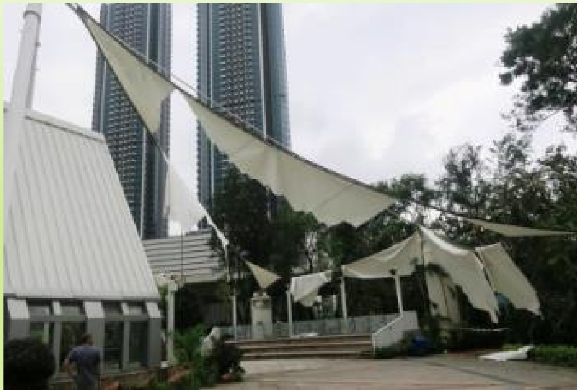
Canopy of amphitheater was torn apart 露天劇場帳篷損毀
