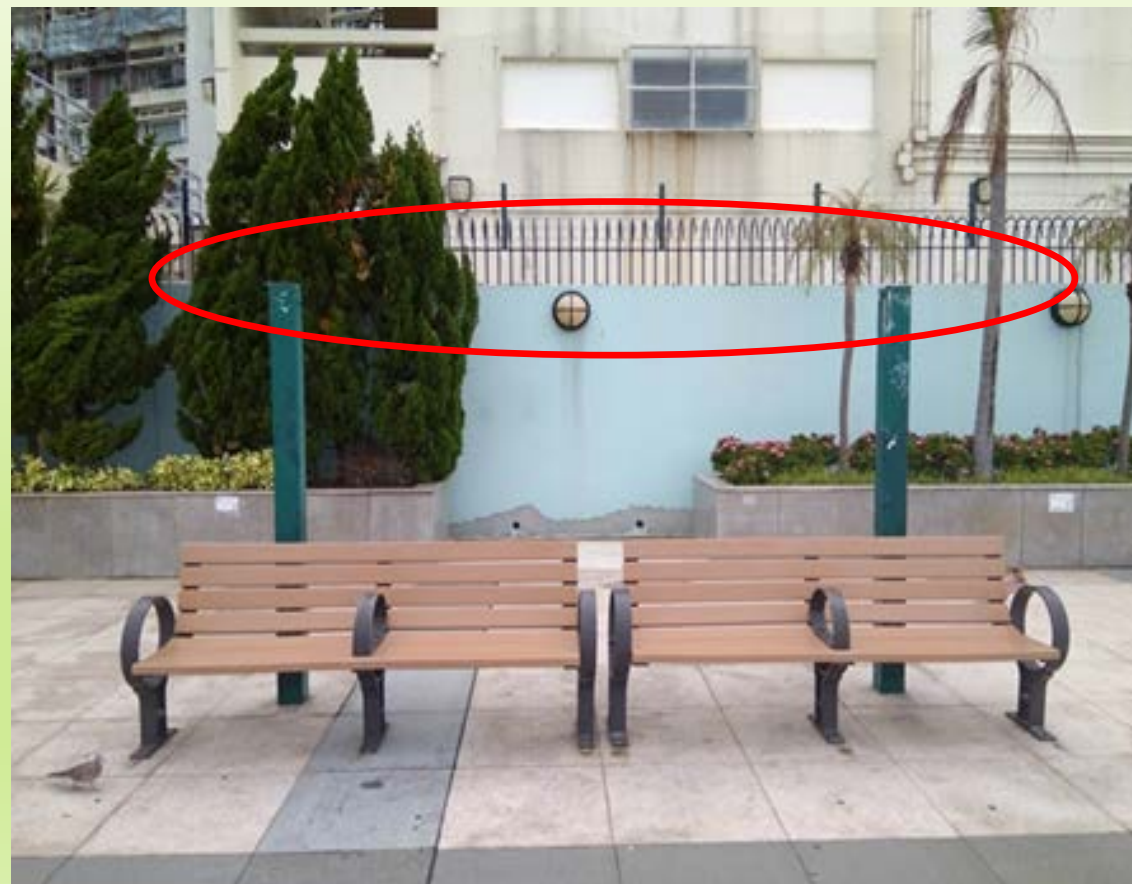
Arbours were damaged 蔭棚損毀
