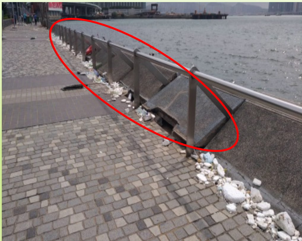
Spalling concrete parapet wall 護牆石屎剝落
