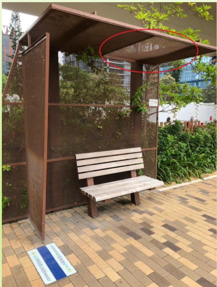
Polycarbonate covers damaged 塑料上蓋損毀
