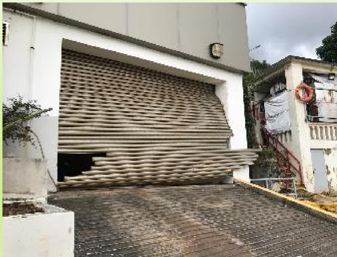
Roller shutter gate was damaged 捲閘損毀
