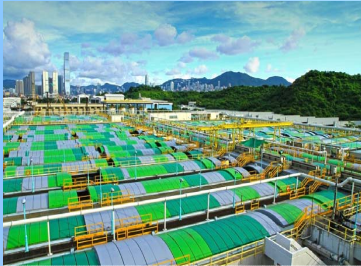
Most Efficient Use of Land for providing a Chemically Enhanced Primary Treatment Plant
