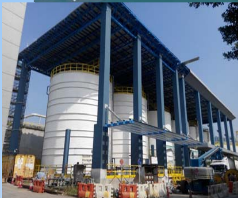
Sodium Hypochlorite Storage Tanks at SCISTW
