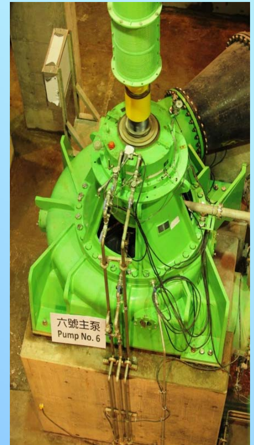
World's Most Powerful Sewage Pumping System in a Chemically Enhanced Primary Treatment Plant
