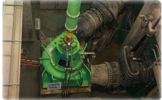
Figure 9 – Pump No.7 inside MPS2
