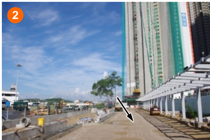
A Planned Pedestrian Walkway leading to Nam Cheong MTR Station (Under Construction)
