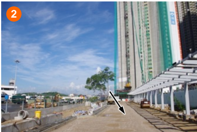
A Planned Pedestrian Walkway leading to Nam Cheong MTR Station (Under Construction)
