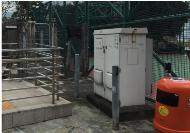
PCCW Cable Cabinet
