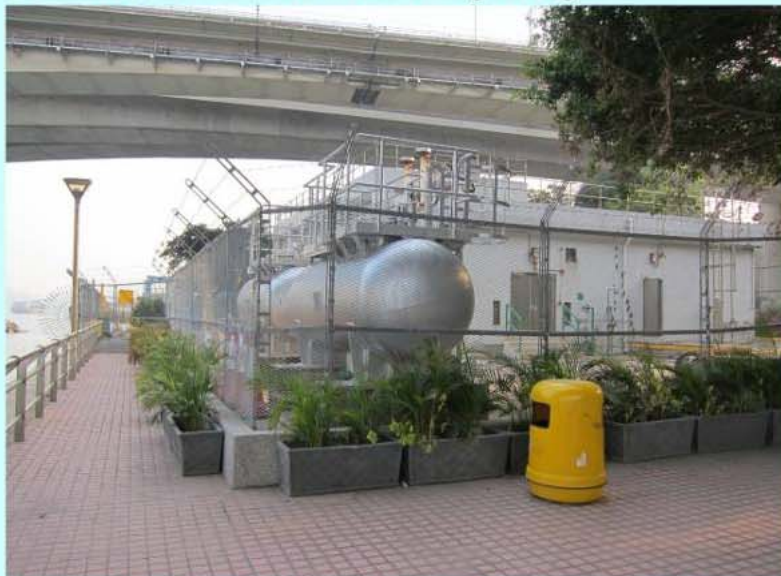
Photo 10: Tsing Yi Salt Water Pumping Station.
