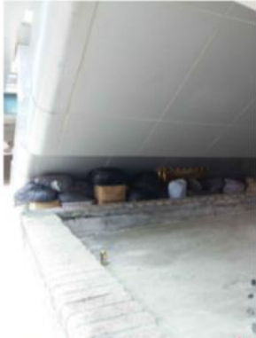
Existing Footbridge: Issues with security and safety concerns
