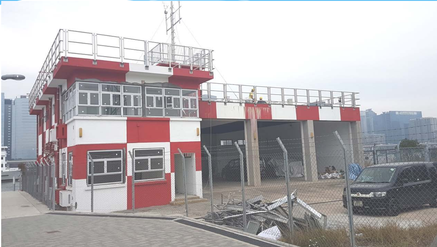
Former fire station building under maintenance and repair by Government in March 2017
