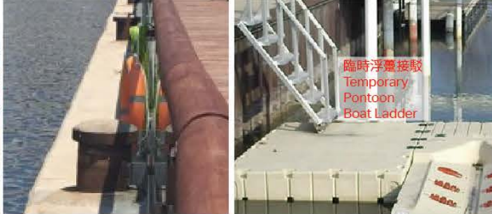
2 可考慮修改繫船柱旁的玻璃欄杆 Proposed Modification of Glass Balustrade along Existing Bollards
