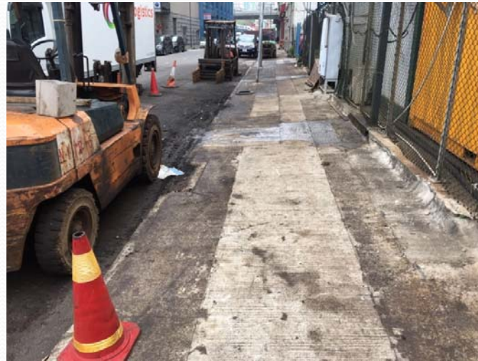
Current condition of footpath at Kai Hing Road
