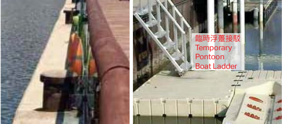
2 可考慮修改繫船柱旁的玻璃欄杆 Proposed Modification of Glass Balustrade along Existing Bollards
