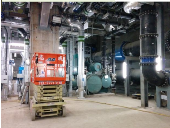
South Plant chillers
