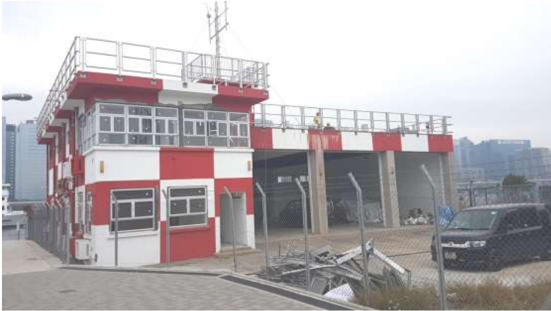
Annex 4: Former fire station building under maintenance and repair by Government in March 2017.
