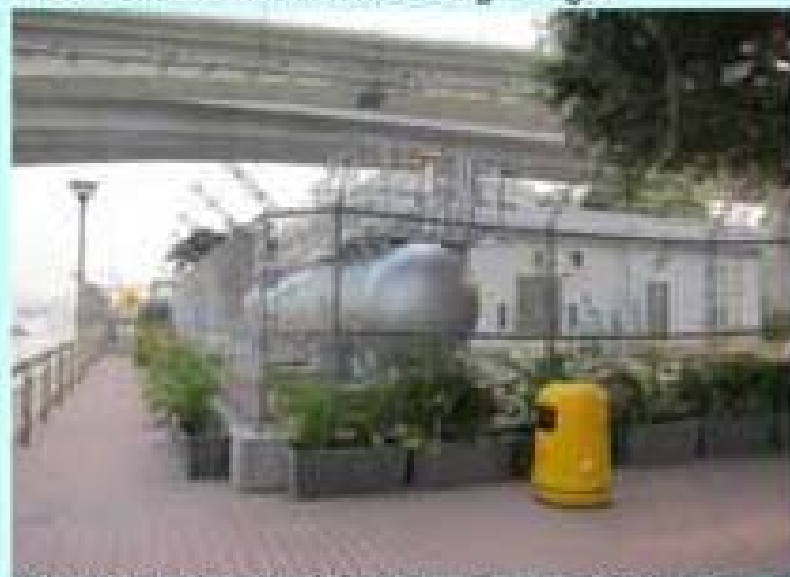
Photo 10: Tsing Yi Salt Water Pumping Station.
