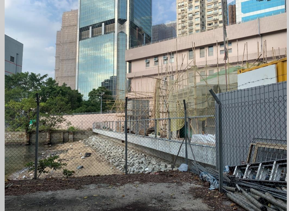
Tin Hau Temple under construction [By Tin Hau Temple Development (三角天后平安堂有限公司)]
