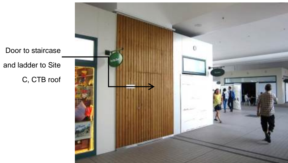
Photo 9: Door to staircase and ladder to CTB roof platforms for maintenance
