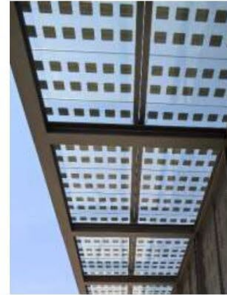
BIPV PANEL ABOVE SHELTERS
