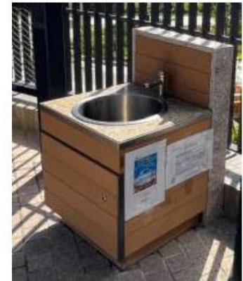
HAND WASHING FACILITY
