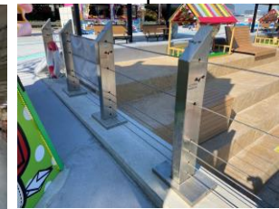
Bollard with Cables
